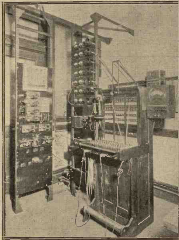
The Switchboard for line connections for "outside broadcasts" at WJZ-WJY.
