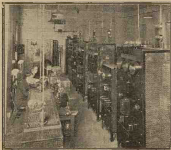
The apparatus room on the roof of WJZ-WJY, New York.
